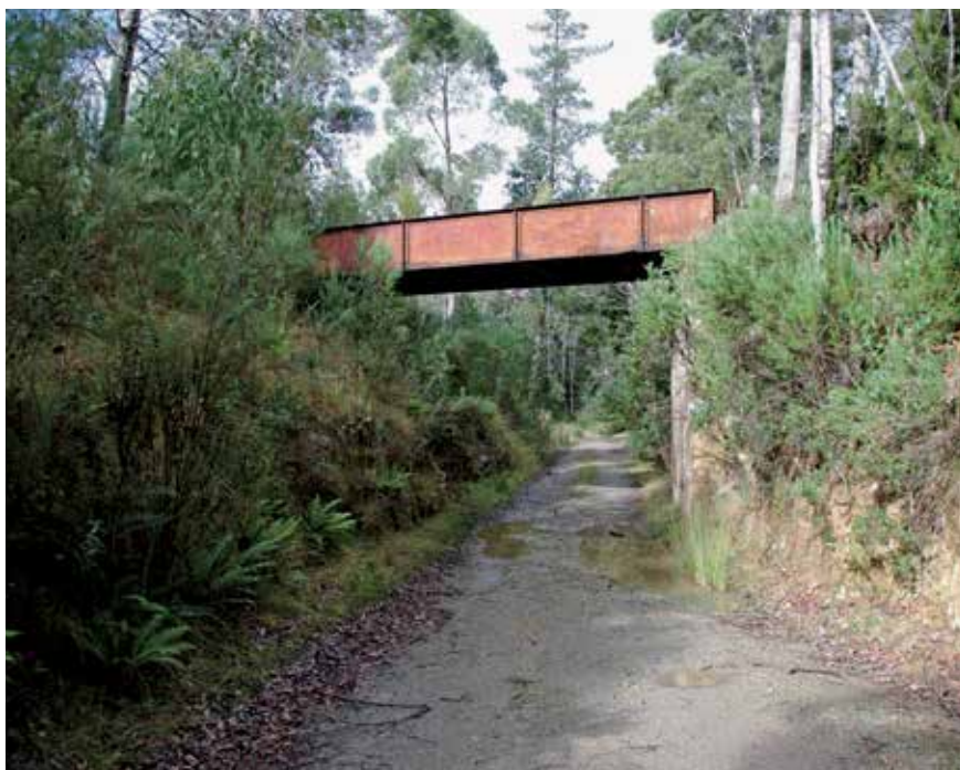
The bridge that took the Emu Bay Railway across the North East Dundas Tramway remains relatively intact, despite not having carried a train for nearly half a century. Photo: Scott Gould
