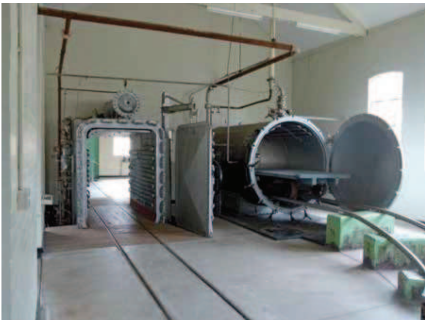
The two autoclaves. A small wooden-framed trolley sits inside the circular unit Photo: Andrew Forbes
