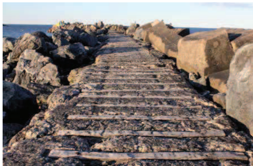
The remains of the Coffs Harbour breakwater tramway, last used in 1974 and soon to be covered forever as reconstruction works raise the wall level, seen on 25 August 2012 Photo: Ken Littlefair
